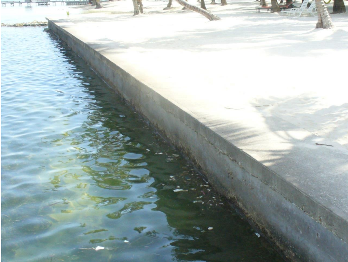
Figure 7.32: Loss of beach area for swimming due to the construction of hard structures (sea walls) in San Pedro, Ambergris Caye
